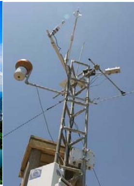
Urban CO 2 Monitoring Station
